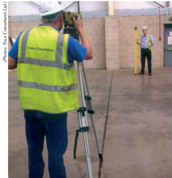
Figure 1: Checking compliance with Property IV limits using engineer's precise level, ppm and invar staff.
