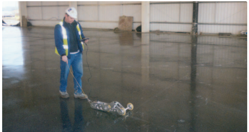
Figure 2: Checking Property II limits with the Face Prop II meter.
