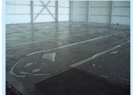
A complete slab covered with water, plastic and a curing compound immediately after casting. This slowed the curing process of the concrete down, reducing the potential for shrinkage cracking.
