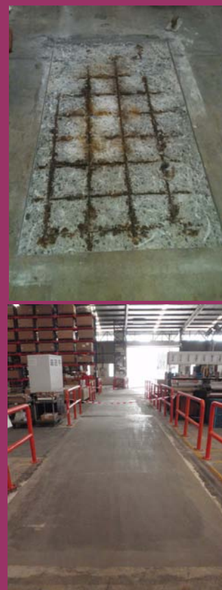
Top: Delamination due to corrosion of rebar; Below: completed floor repair
