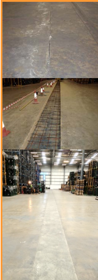
From top: Damaged floor joints; Clean arris edges with dowel bars installed; Completed floor joint repairs
