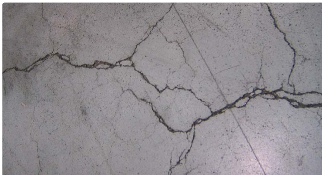
Figure 1 top: Excessive cracking in a conventionally reinforced floor.
