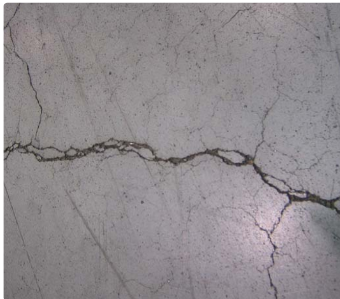
Figure 4: Breakdown of surface at cracks
